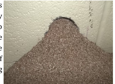
Figure 4: Loose insulation spilling out of a hole in an exterior concrete block wall.
